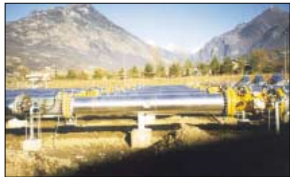
Six run energy system 2,300,000 m 3 /h at 60 bar
