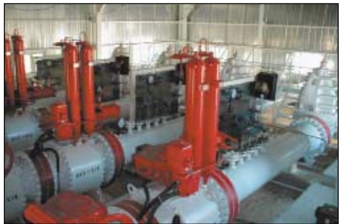
Border metering 1,200,000 m 3 /h at 75 bar
