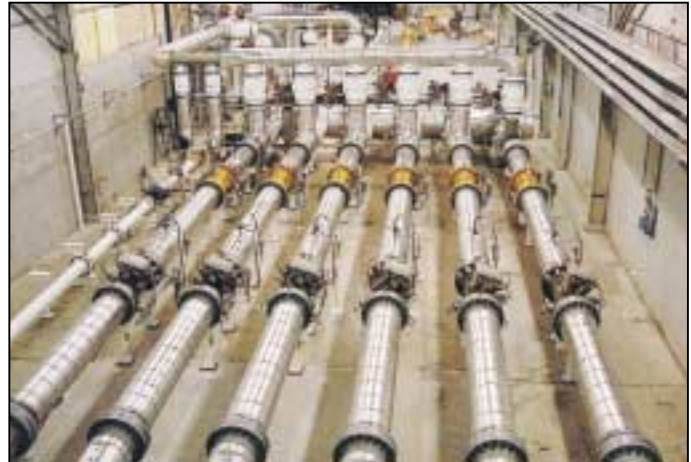
High pressure calibration facility Winnipeg
