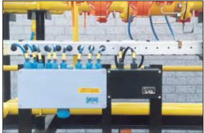
Electrical and instrumentation engineering
