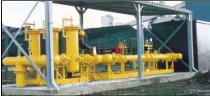
Gas measurement system
